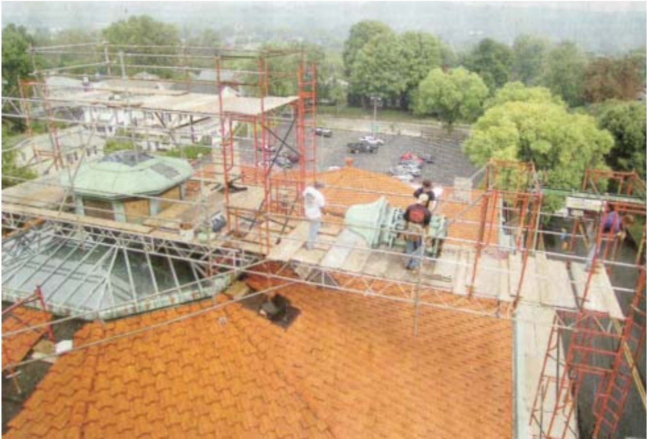
Seen from the bell tower above, workers from The Durable Slate Co. move across a system of scaffolding above pedestrians and automobiles passing by High Street as the workers remove the original cupola from the roof of First United Methodist Church on Thursday. (E-G photos by Ken Ritchie)
