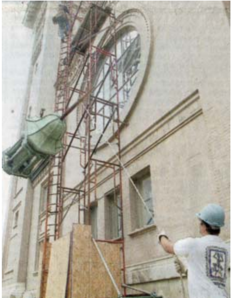
Ron Ladina, 40, of The Durable Slate Co. in Columbus, uses a rope to guide the First United Methodist Church cupola away from a large stained glass window during its descent from atop the church.
