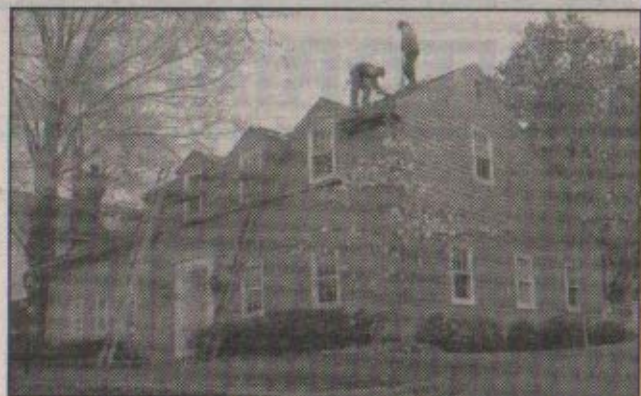
Carol Note's house at 126 E. Columbus St. in Canal Winchester receives roofwork from a Durable Slate Company crew.
